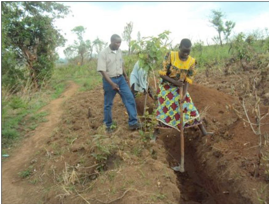
Erosion canal-digging activities under the supervision of an LWF extension officer in Gashirwe colline just above Rumpungwe marches.
